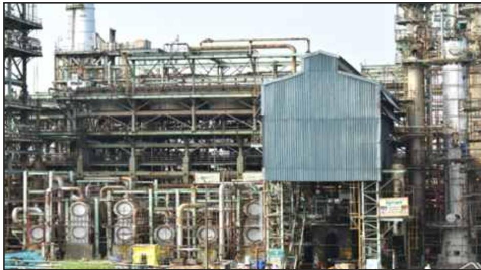
DHDT Revamp completed & commissioned on 22.11.2019 at Chennai
