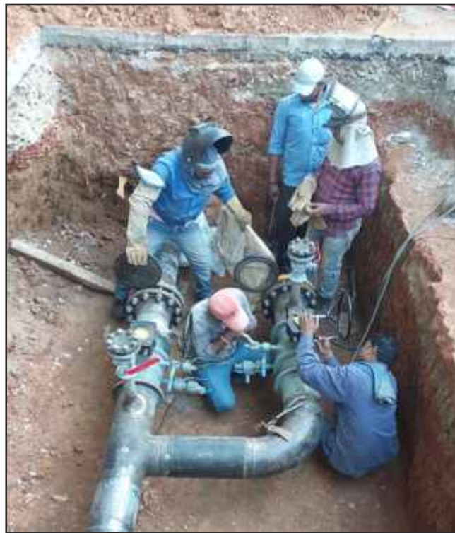
Intel Connectivity, CGD Project, Bengaluru
