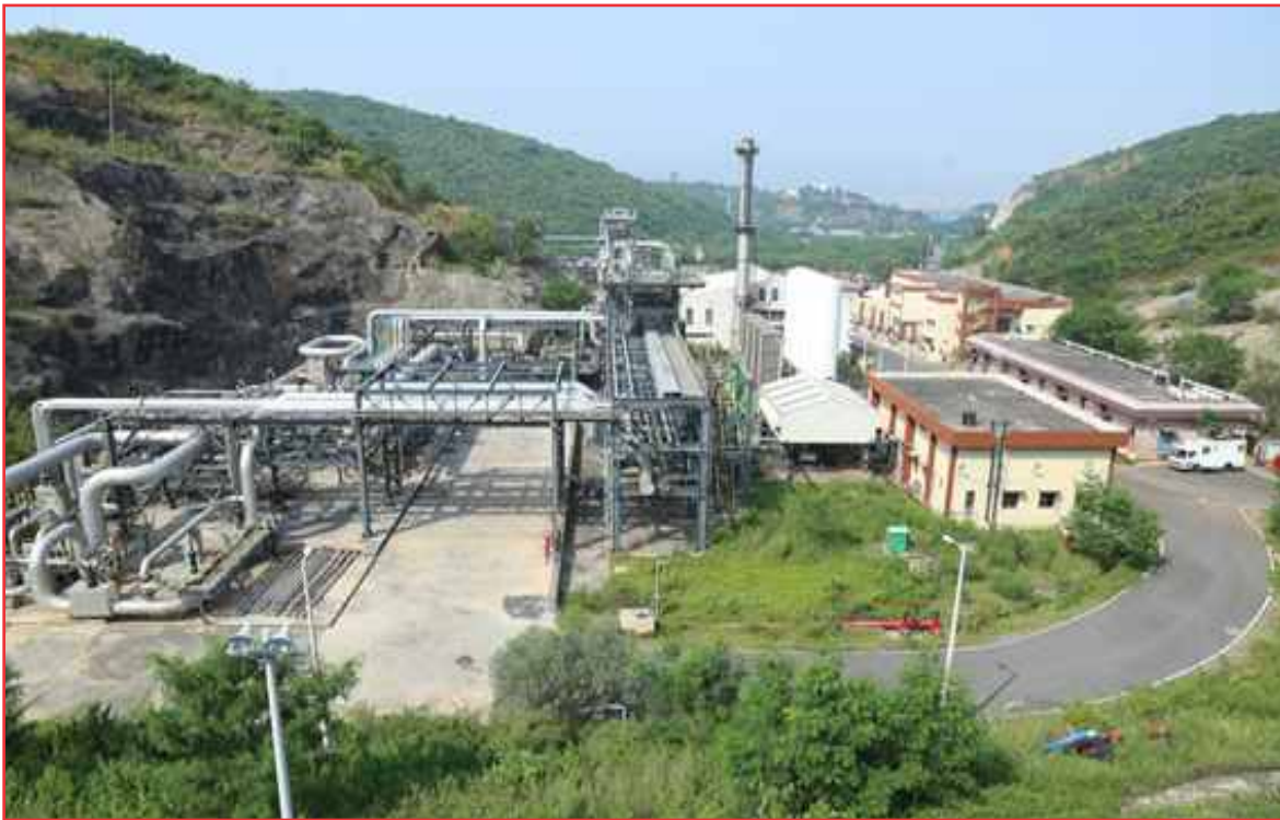
View of the aboveground facilities at Visakhapatnam
