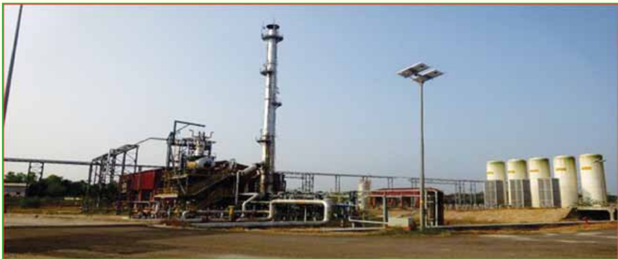
Flare area of Padur Facility
